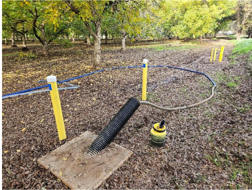
Photograph 11. Discharge line from irrigation well going into reverse tile drain system.
